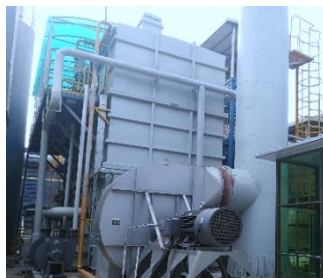
RTO Environmental Protection System in Huizhou Factory
