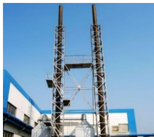
Dust Treatment System in Suzhou Factory
