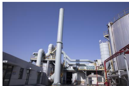
RTO Environmental Protection System in Tianjin Factory
